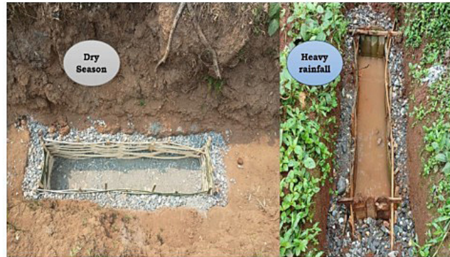
Fig. 8: Recharge pit installed in TRA Nagrakata research plot" and introduces the concept of Recharge Shafts.
